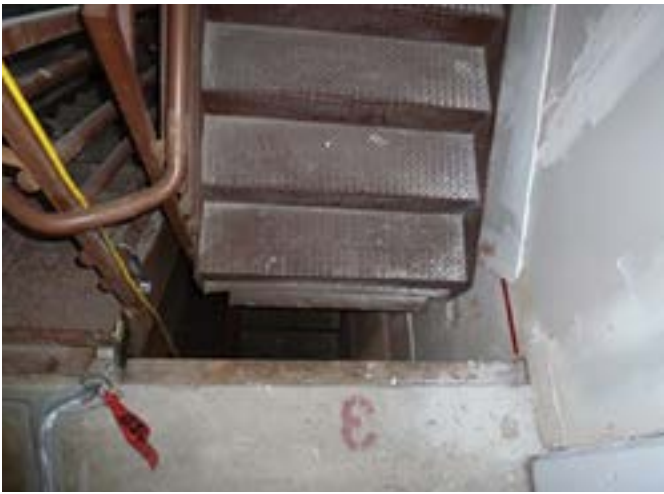
Damage to stair system from 5-story specimen earthquake test. Photo credit - Pantoli et al., 2013
