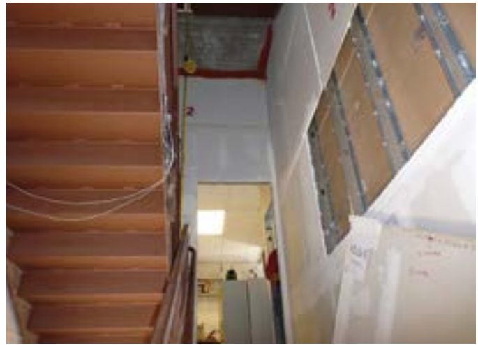
Damage to fire compartment barrier from 5-story specimen earthquake test. Photo credit - Pantoli et al., 2013
